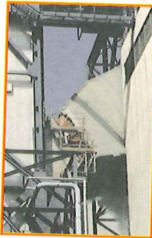
Installation in a DeNOx-plant
